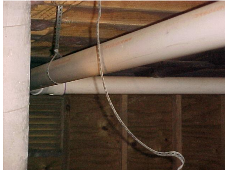
Broken metal retaining strap at PVC drain line in sub area.
