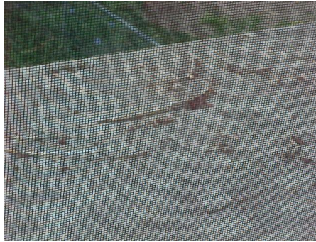
Debris should be removed from the roofing in various locations, e.g. front.
