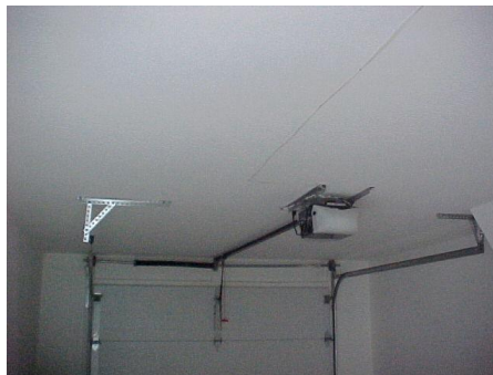
No attic access hatches at detached garages (very small attic areas).
